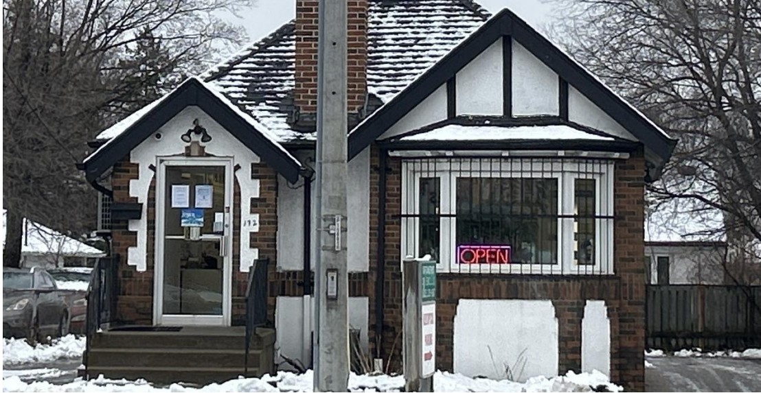
Photo 15 Example of inappropriate alteration to historic entrance feature where original arch shape has been altered with rectangular glass door
