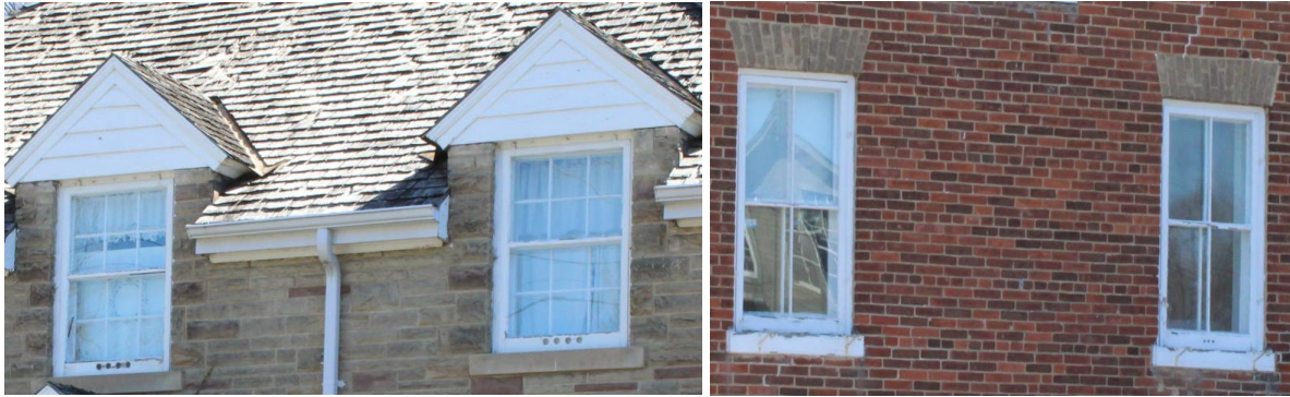
Photo 10 Examples of historic wood windows in the HCD, shown is 6/6 and 2/2 windows
