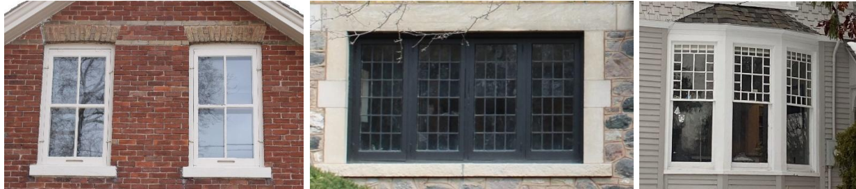
Photo 11 Examples of historic windows in the HCD including 2/2 wood sash, multi-pane casement, and bay windows
