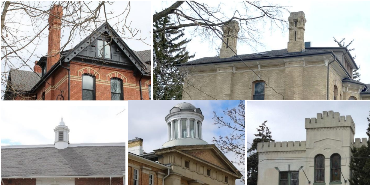
Photo 1 Examples of character defining roof features in the HCD from top left to bottom right including brick chimneys, eaves, cupolas, and parapet battlements (see Appendix C for Architectural Terminology)
