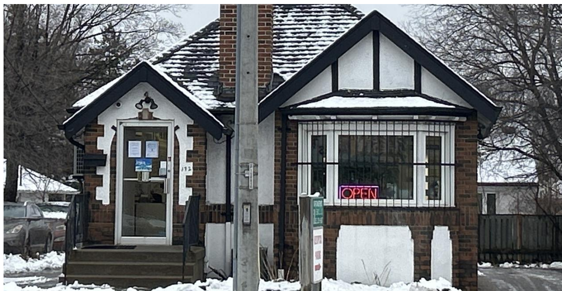
Photo 14 Example of inappropriate alteration to historic entrance feature where original arch shape has been altered with rectangular glass door
