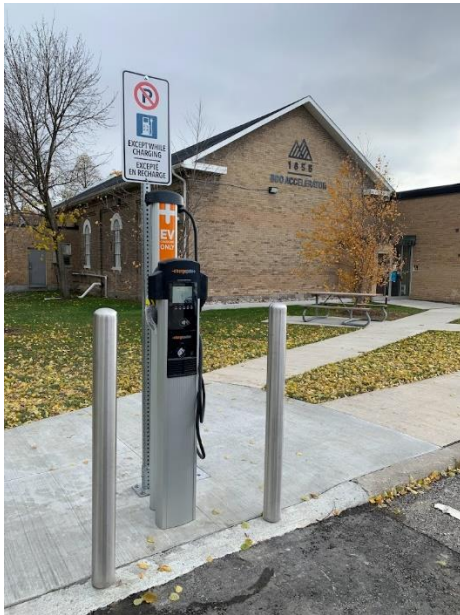
Figure 9 Level 2 EV Station at 1855
