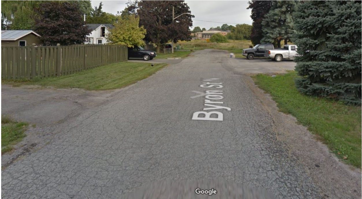
Figure 14 A photo of a road in Very Poor condition
