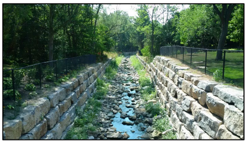
Example of armour stone used to line the banks of open portion of the channel
