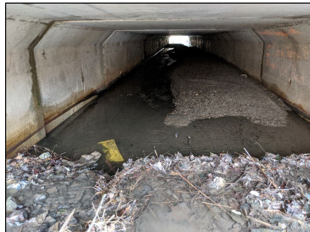
Sediment accumulation with Victoria Street West culvert crossing
